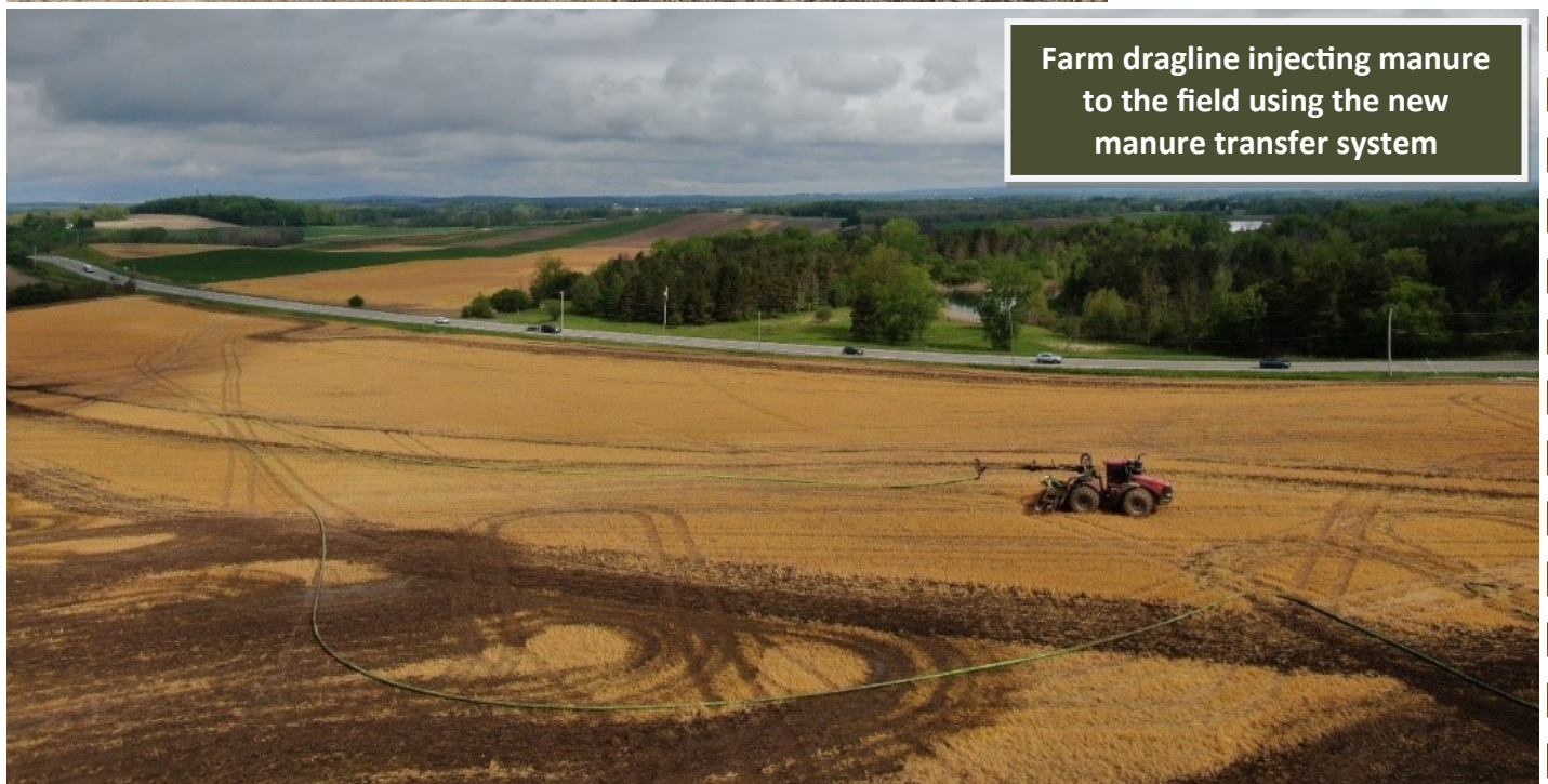
New waste transfer under NYS Rt 5&20 after construction with operational dragline connected to the new transfer pipe
